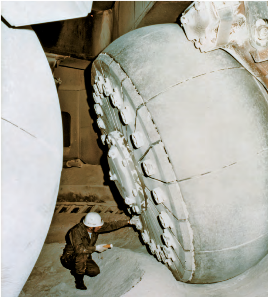
1 | 2 Inside and outside views of the biggest vertical mill in the world at that time, an MPS 4850 A supplied by Gebr. Pfeiffer to Japan in 1976.
