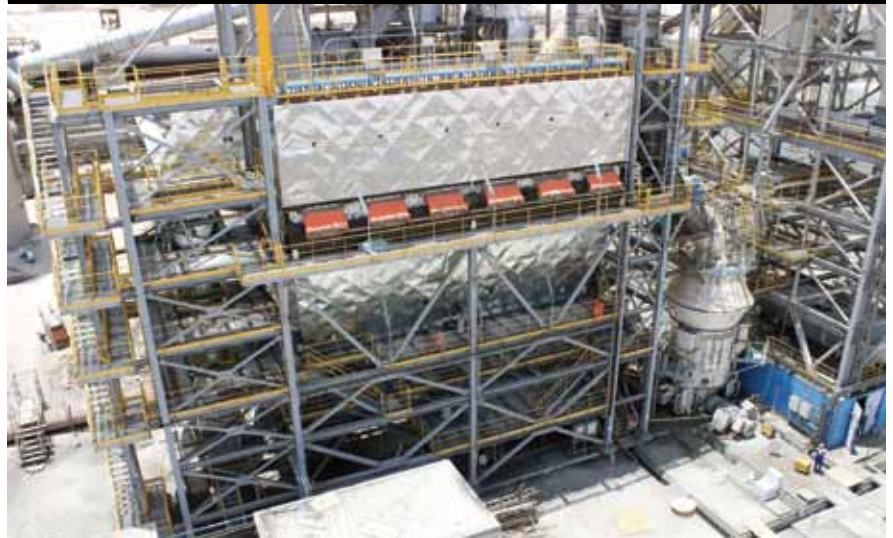
Figure 1: the grinding area at BMIC's Assiut plant includes an MPS 2800 BK VRM and process filter with flow volume of 160,000m 3 /h
