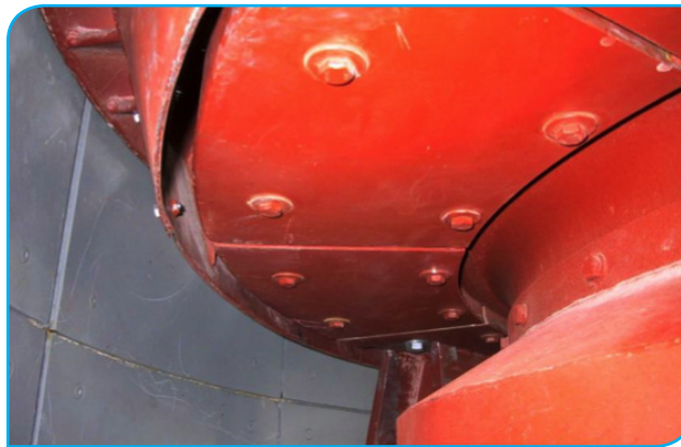
Left - Figure 3: Heat shield and thermal insulation for grinding bowl in hot gas channel.
