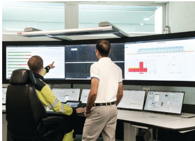
ABB Ability Expert Optimizer is an advanced process control solution used to help cement producers reduce their carbon emissions. Photo: ABB
